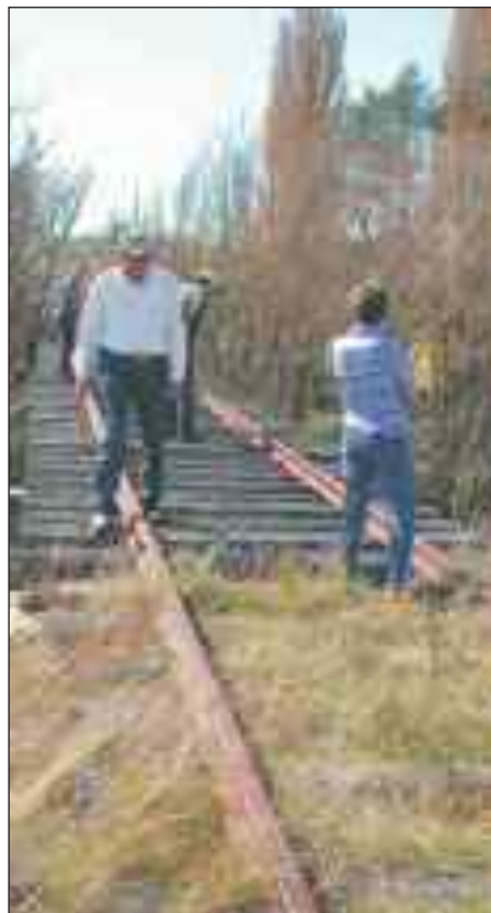
OTHR members inspected the wooden trestle bridge over Snakes Valley Creek recently.
